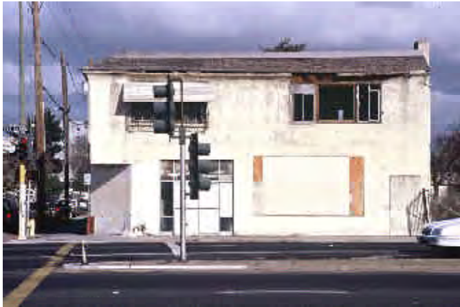
This structure at Auzerais/Bird has been a neighborhood eyesore for years. It will soon be demolished for new development.
